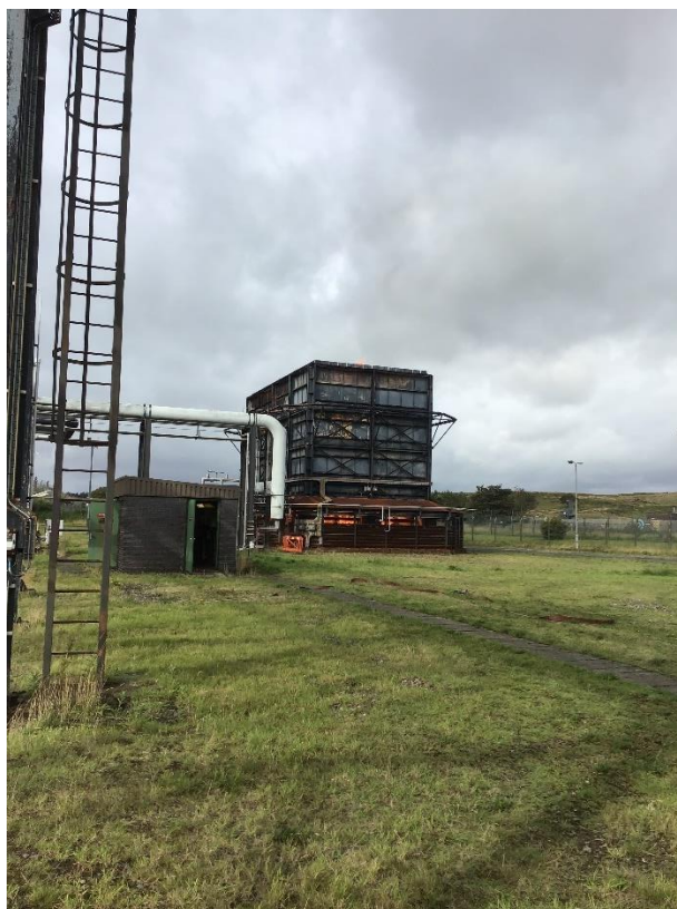
Photo 1: Photo of one of the Ground flares at the Shell UK site.
